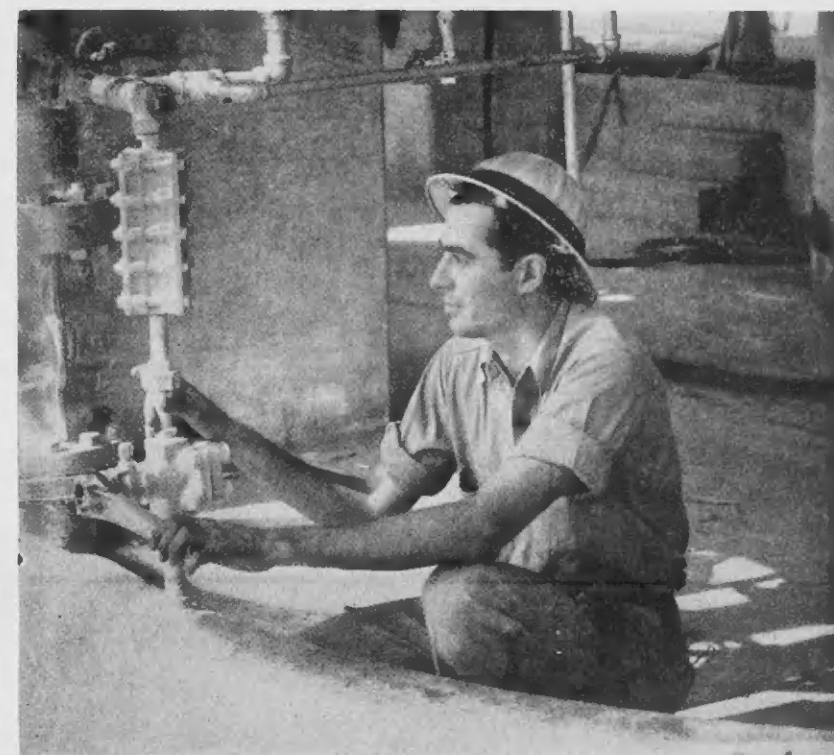
A FLS. 400 supplemental award goes to W. de Souza for his idea which has already won an initial Fls. 100 and a capital Fls. 400. His idea was to install a sight glass in catalyst loading line from 1/2 ton hopper.
